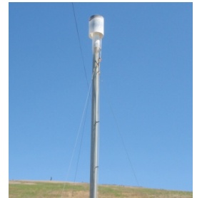
Flares incinerate odorous gases
