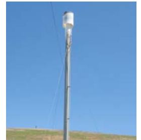
Flares incinerate odorous gases
